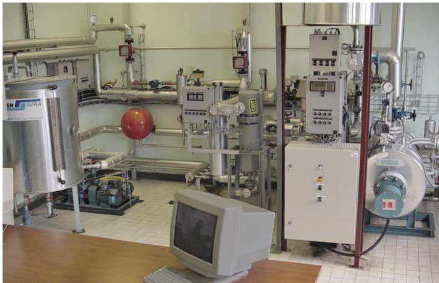
Fig. 10.49. General view of the steam generator
